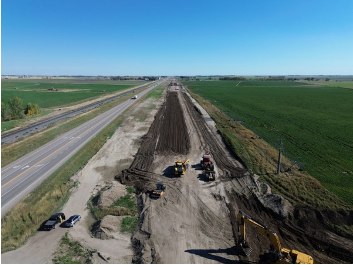
Subgrade Disking and Compacting Prior to Gravel Placement at RR 160 Facing East
