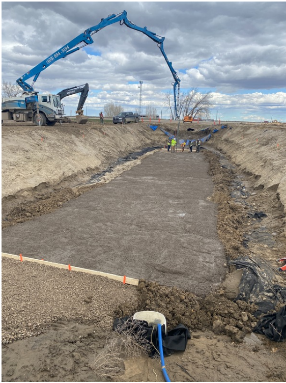
Pouring Concrete Slab on Structure 6 Due to High Ground Water Table South of Purple Springs Facing North
