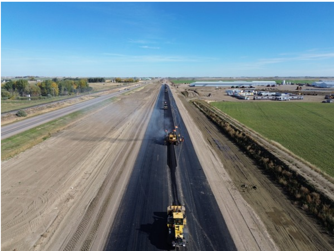
Tack Oil and First Lift of Asphalt Between RR 162 and 161 Facing East
