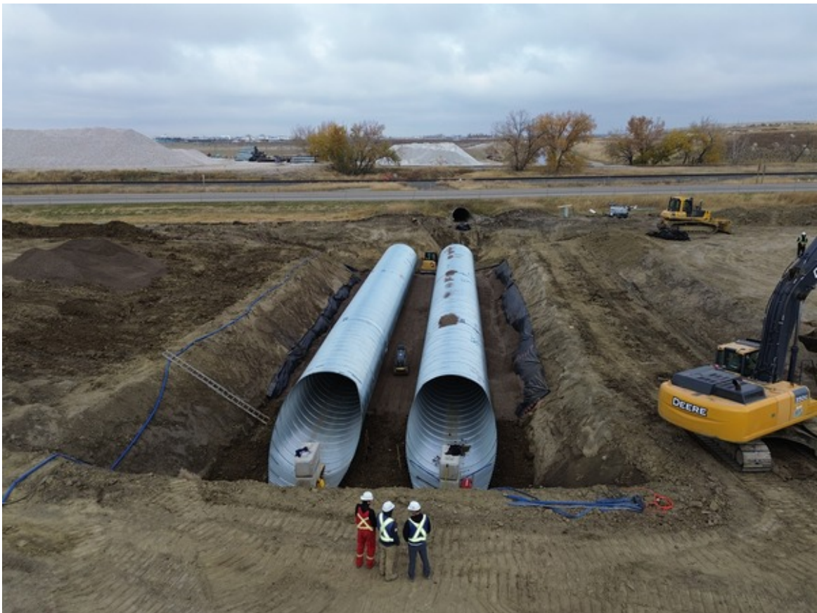
Bridge Structure 1-2 Under East Bound Lane Between Taber and RR 163 Facing North
