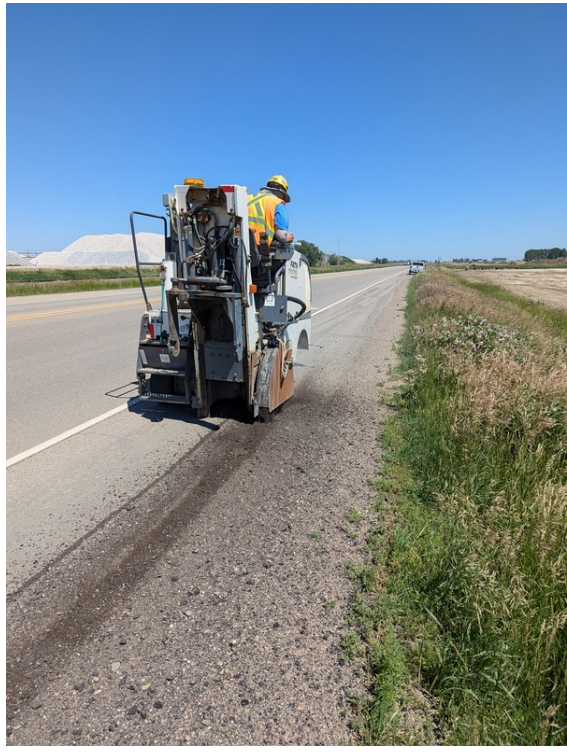
Saw Cutting and Removing Field Access Between Taber and RR 163 Facing East
