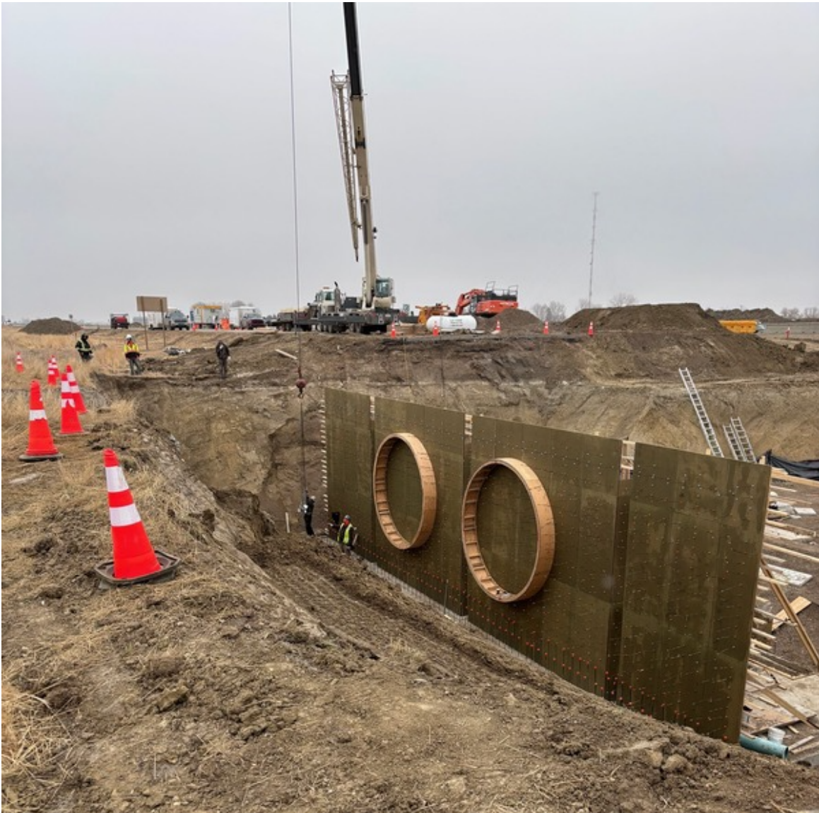
Placing Circular Forms and Rebar on Headwall of Structure 1-2 Between Taber and RR 163
