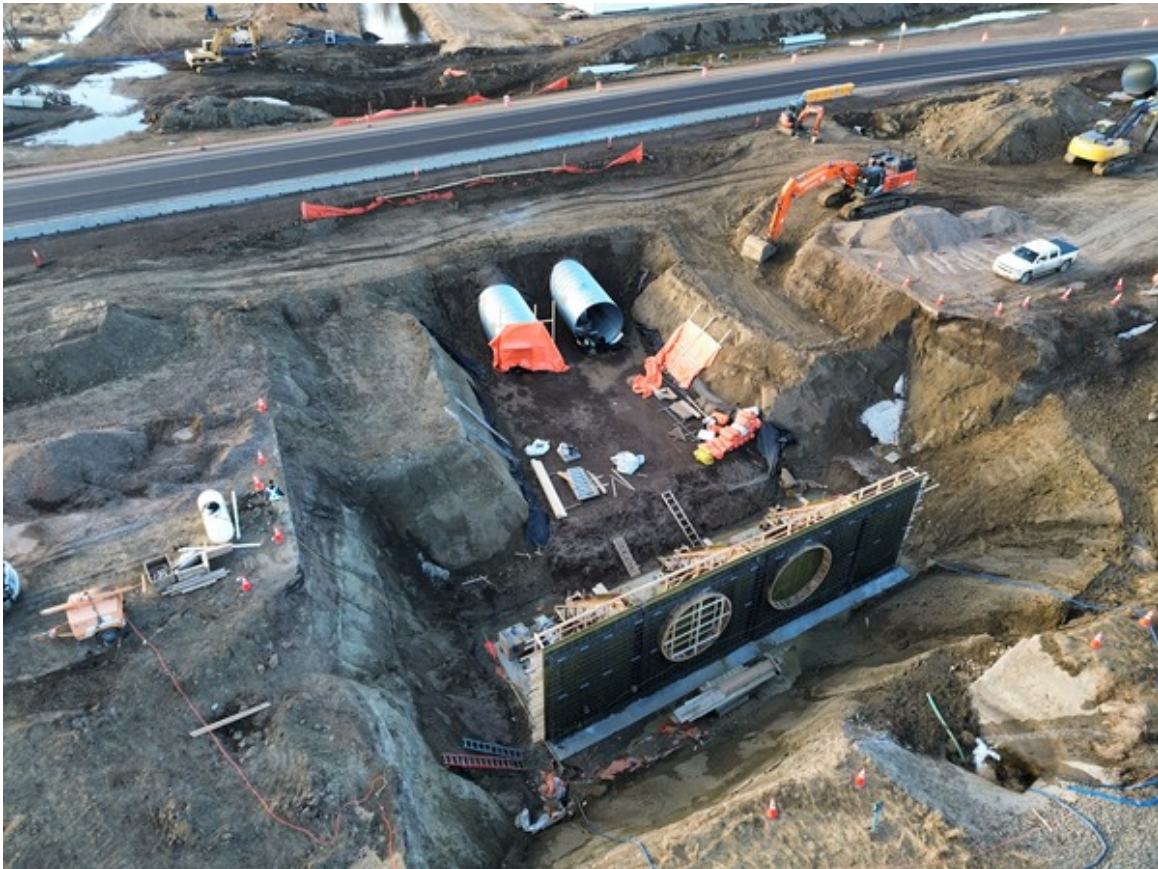
Placing Form Work and Installing Rebar on Structure 1-2 Between Taber and RR 163
