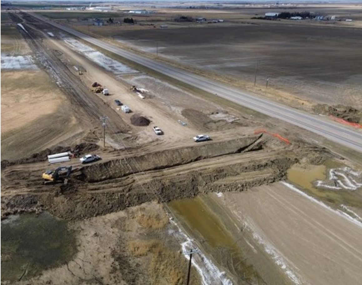
Completing Bore Under Existing Highway at Lateral 8 East Horsefly Between RR 152 and 151
